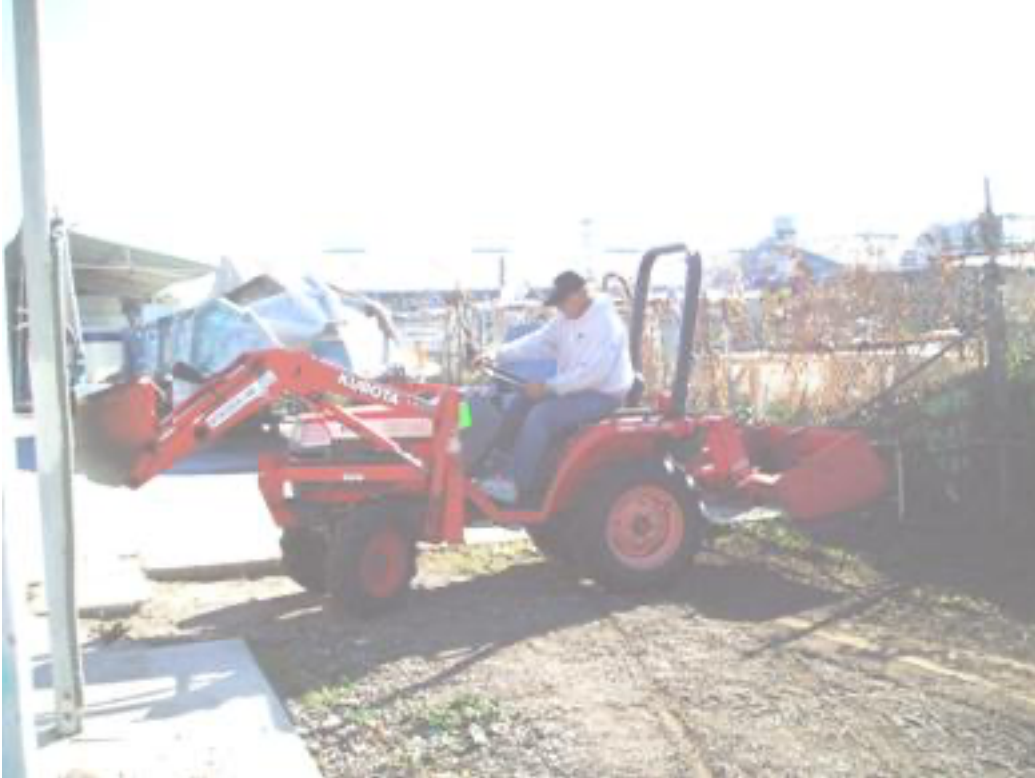
Don gets in touch with his inner farmer -grading the dirt to get ready to lay the cement
