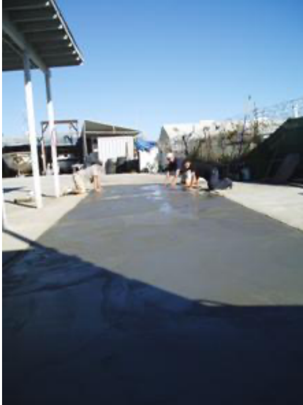
Boat builders become cement masons! Matt (left), Don and Oscar finish up the cement in one of the last remaining dirt areas
