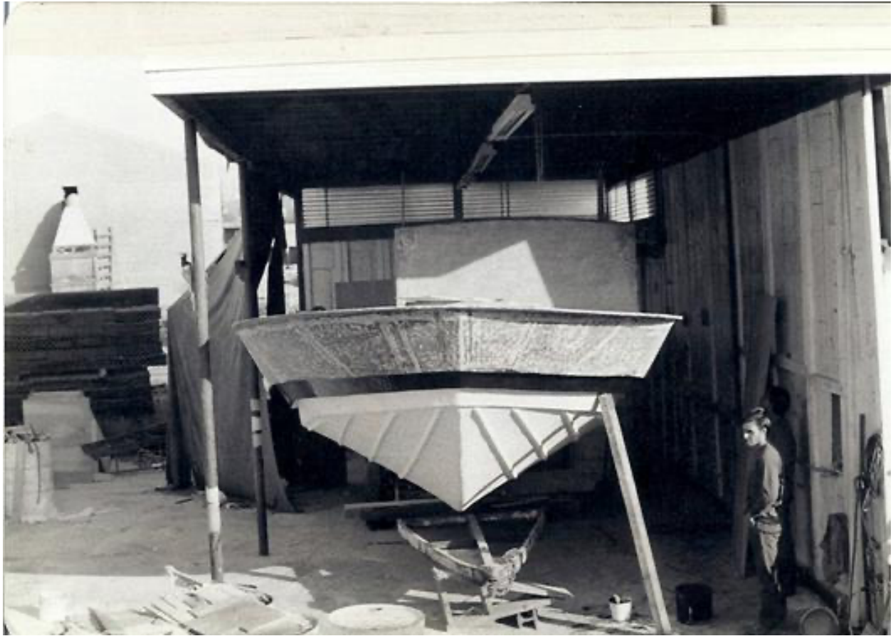
Early '70's - a wooden 36' Radon under construction at the Santa Barbara Street boat yard
